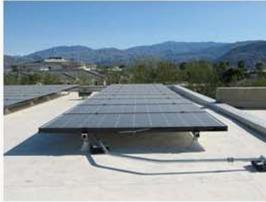
HeliPower solar installation in Rancho Mirage, CA
